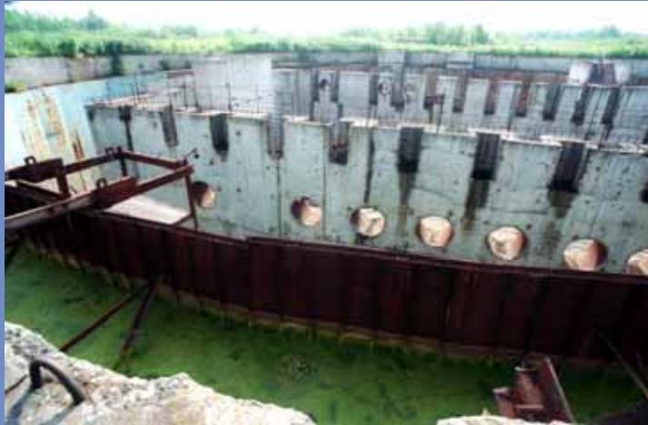
SWTP main pumping station in 2002
